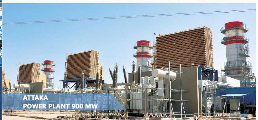
BANHA POWER PLANT 750 MW
